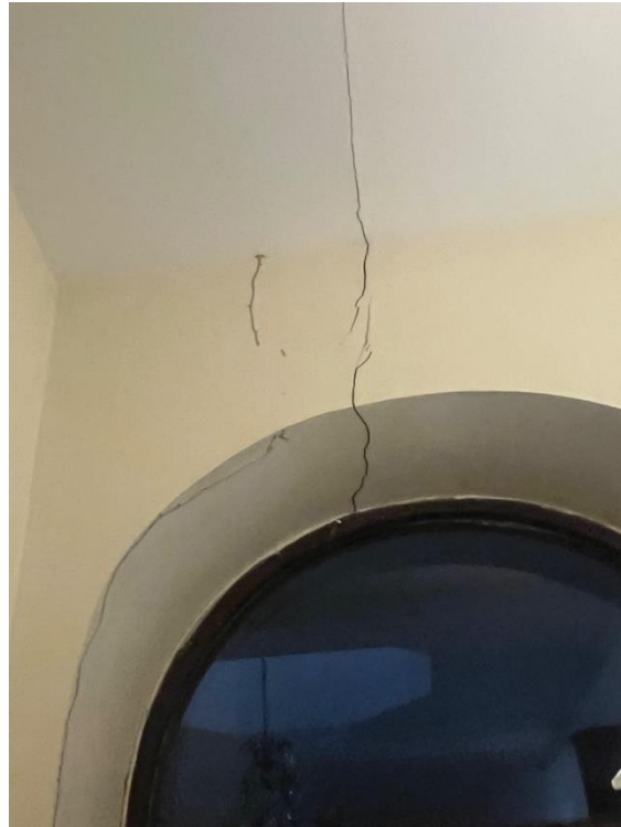
Fig. 1-4 crack in building body due to foundation displacement
